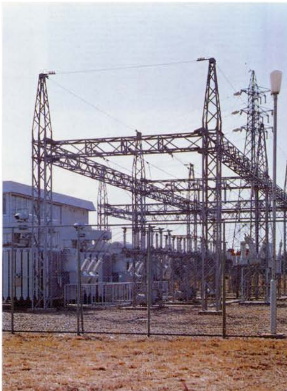
特高受電施設 High voltage power supply.
