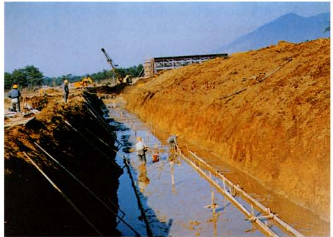
工作棟前の共同溝工事 Construction of an underground tunnel in front of the main workshop.
